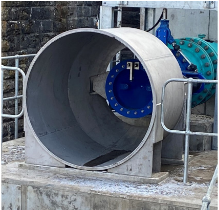
The discharge valve with the bespoke hood, which is secured to the concrete floor.
